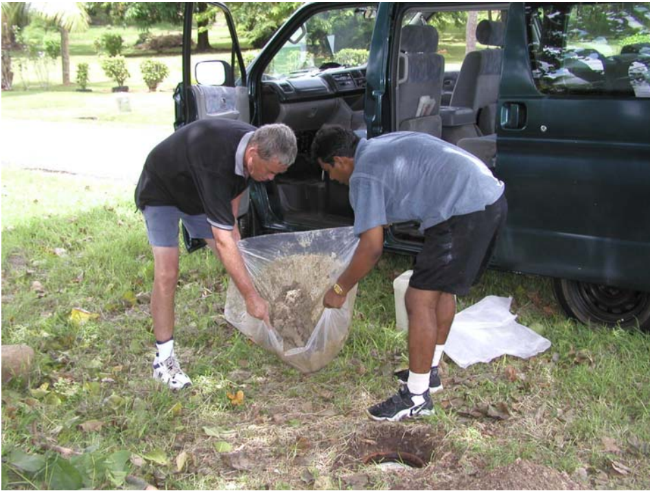
Brian Ratcliff and Andrick Lal mixing concrete in a plastic sheet to establish a new benchmark in the FSC compound in Lautoka, Fiji Islands.
