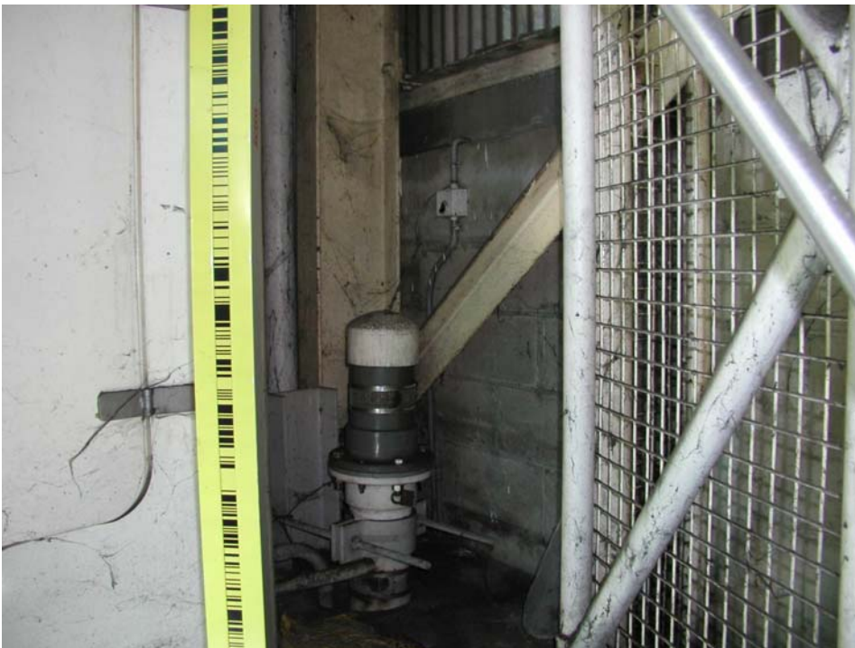
The NTF Tide Gauge stationed in the Ports Authority shed in Lautoka, Fiji Islands.
