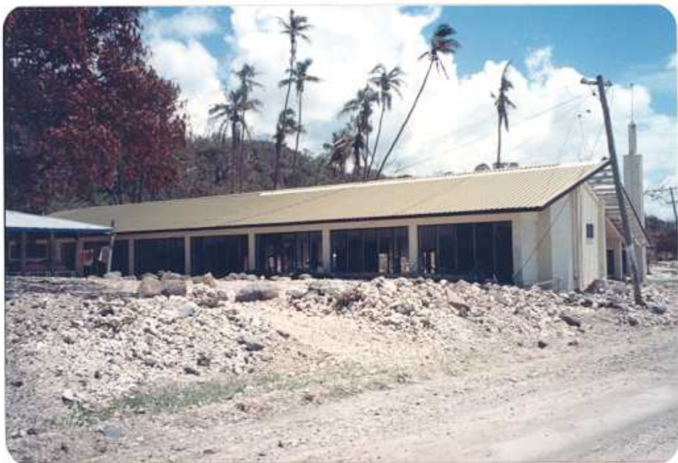
Figure 5. Church at Lautuanuu Village which suffered internal damage from waves and roof damage from high winds. Note the large amount of coral rubble surrounding the church grounds.
