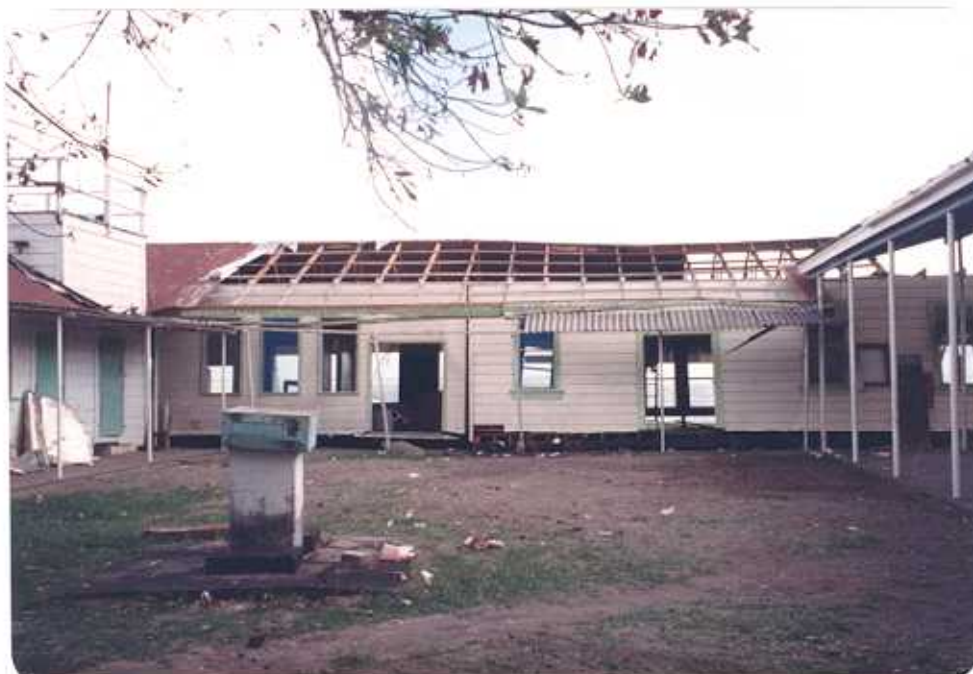
Figure 17. Most of the wooden structures at the Apia Observatory were damaged beyond repair.
