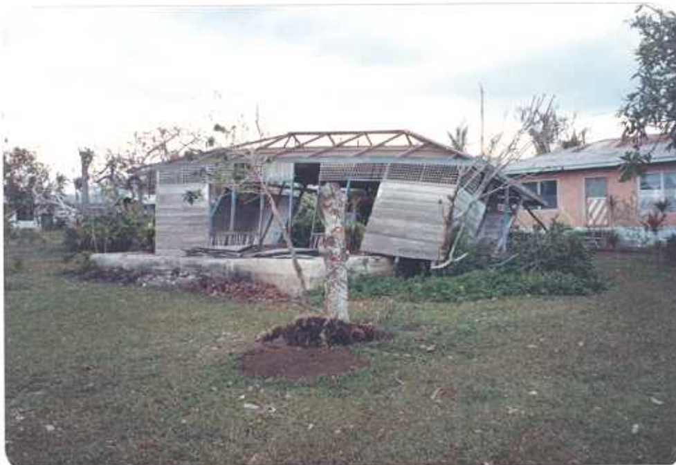
Figure 7. Destroyed house knocked from its foundation by strong winds. The house lies to the west of Apia and is away from the coastline.
