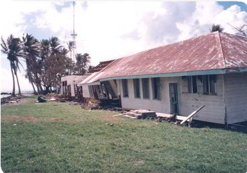
Figure 18. Observatory buildings facing the lagoon felt the full onslaught of the cyclone. Interior, as well as exterior, damage was almost total and the buildings are structurally unsafe for use of any type at present.
