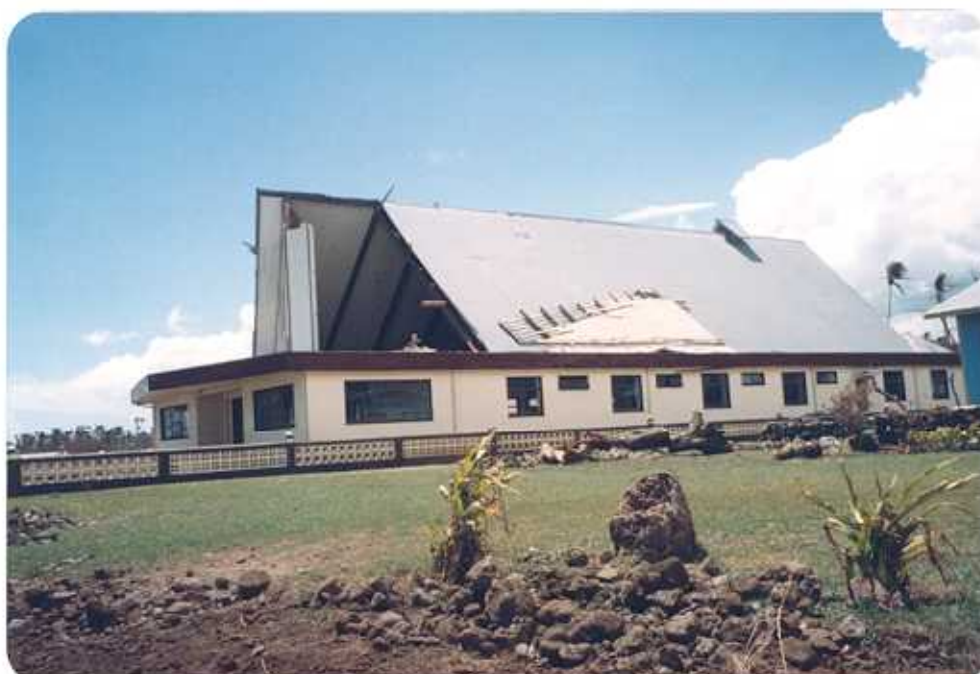
Figure 9. This church at Faleasiu Village suffered damage to its roof. Most structures that lost their roofs also suffered considerable water damage to interior furnishings.
