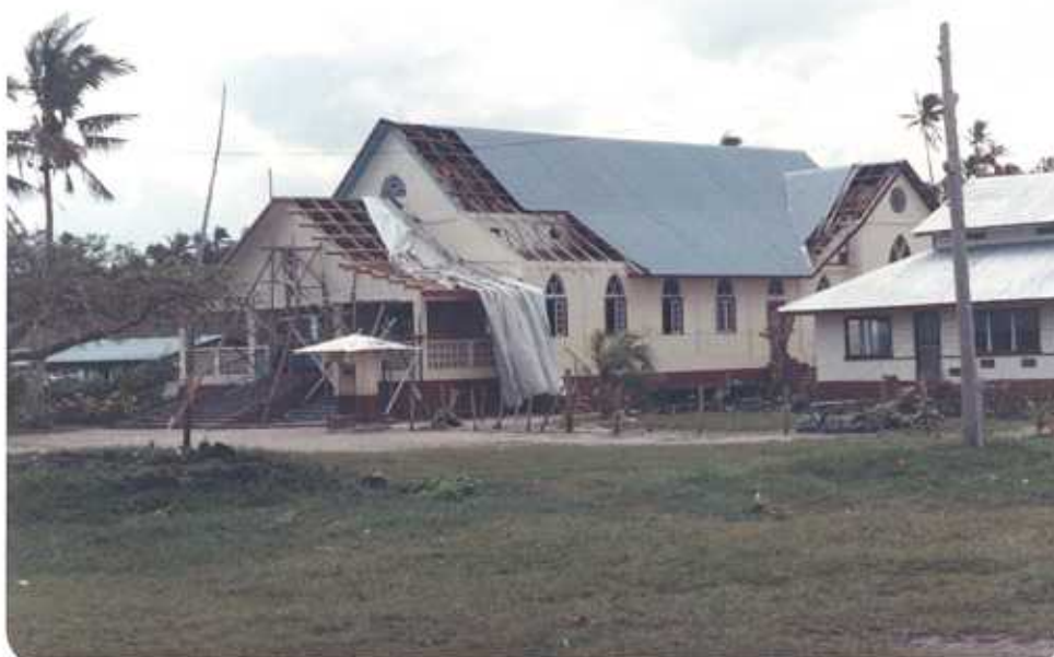
Figure 8. Much of the damage to structures to the west of Apia was caused by strong winds. This church is at Mulifenua Village.
