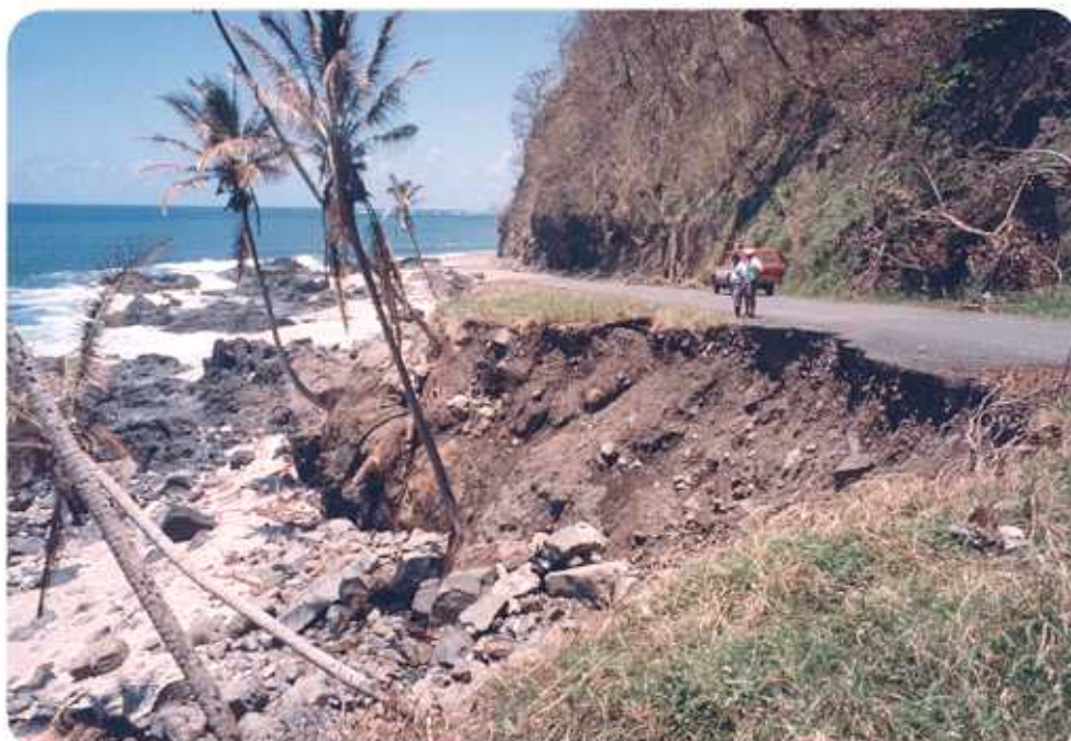
Figure 24. Storm waves to the east of Apia were particularly destructive due to the lack of reef protection in some areas. This photo is of the same area as Figures 2 and 3 and shows the height that storm waves were able to reach during the cyclone.
