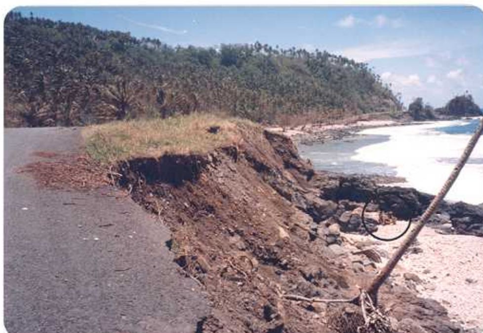
Figure 3. Cliff erosion at edge of road where truck in Figure 2 was washed from road. Truck remains are circled.
