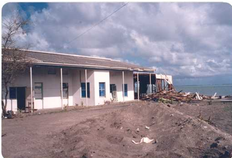
Figure 16. The Apia Observatory suffered considerable damage both to buildings and the effects housed there. A large amount of sand was deposited during the storm on the end and east side of Mulinu'u Peninsula.
