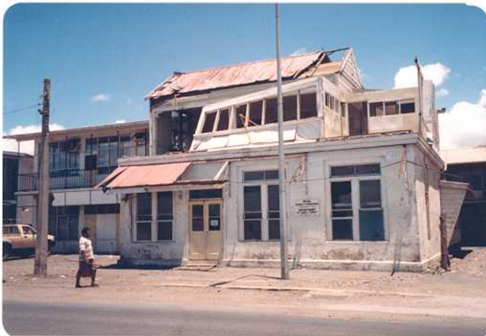
Figure 20. The Department of Lands and Survey building suffered considerable damage. The building lies on the main road fronting the harbour at Apia.
