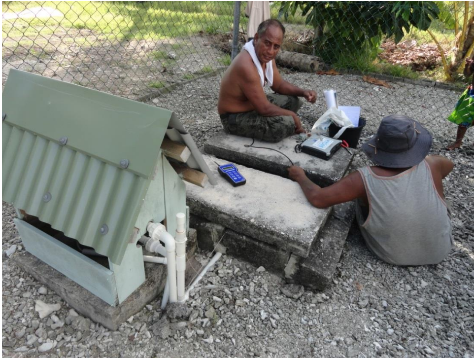
Figure 10. Health Clinic well, which showed brackish water quality, is attached to a solar pump system that was not working during the survey.
