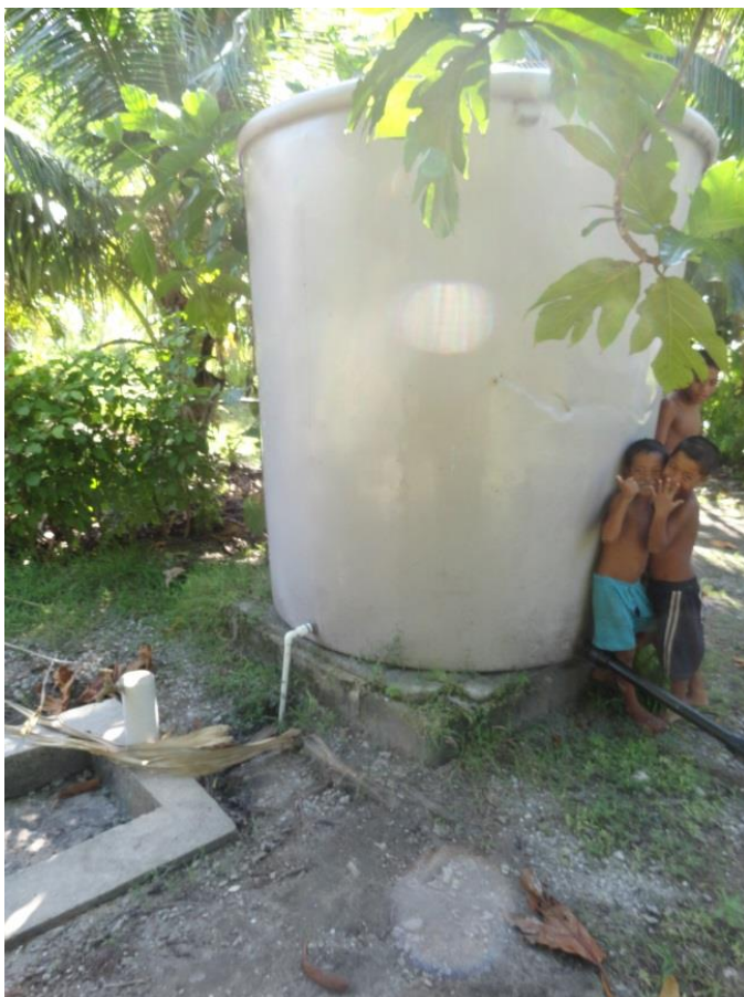
Figure 11. Rainwater tank connected to a tap stand in Kiebu Village.
