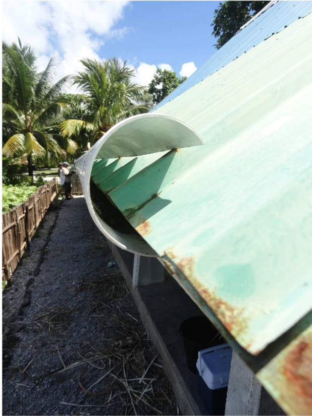
Figure A12-8. Split PVC pipes used as guttering on a maneaba roof catchment – the pipes allow splash losses from the rainwater collection system.
