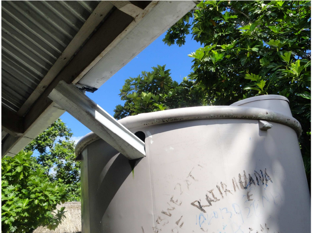
Figure A12-6. Inadequate RWH facility showing the use of an additional gutter as downpipe.
