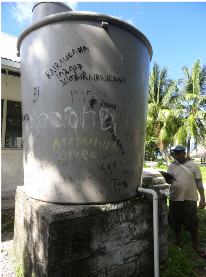
Figure A12-7. Rainwater tank mounted on a raised tank stand.
