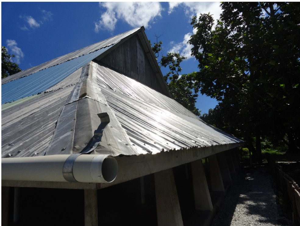
Figure A12-9. Split PVC pipe used as guttering and covering some parts of the roof edge.
