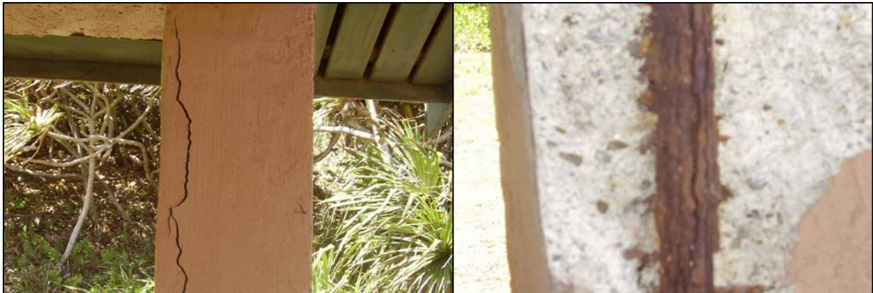
Figure 15. Photos of the concrete post of the SSD rest house. A) Cracking is visible on the post of the rest house. B) Vertical cracks in the corroded metals indicate the expansion of the metals during corrosion that resulted in the cracking of the concrete.
