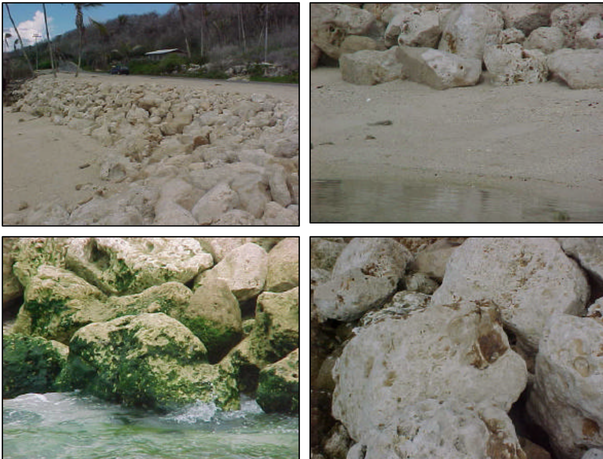
Figure 22. Rip-rap characteristics at the harbour site. Top left – a single-layered rip-rap, protecting an eroded segment of road, on the Southern side of the harbour; top right – rip-rap at the toe of the groin; lower left – algae-covered rip-rap at the toe of the groin, alongside the mooring basin; and lower right – note rip-rap boulder shape, angularity and pits.
