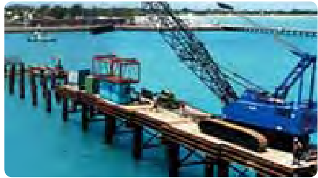
Improving the lifeline of Kiribati: Enabling large ships to berth at Betio Port (source: Japan International Cooperation Agency).
