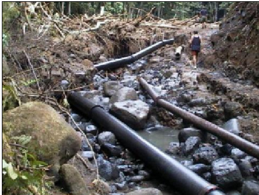
Figure 3.1: Damaged pipeline near Fuluasou River
