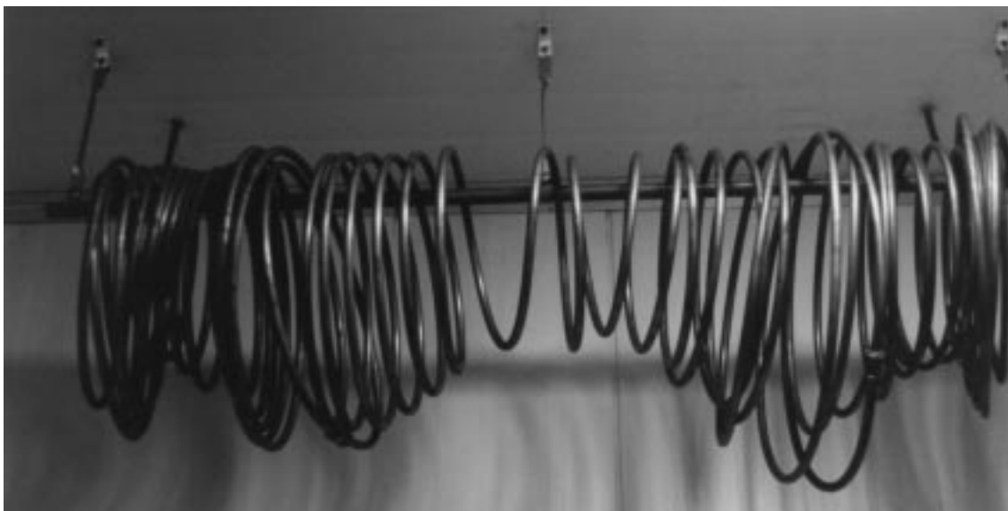
Figure 8: Copper piping mounted in chill room to provide chilled water to processing area
