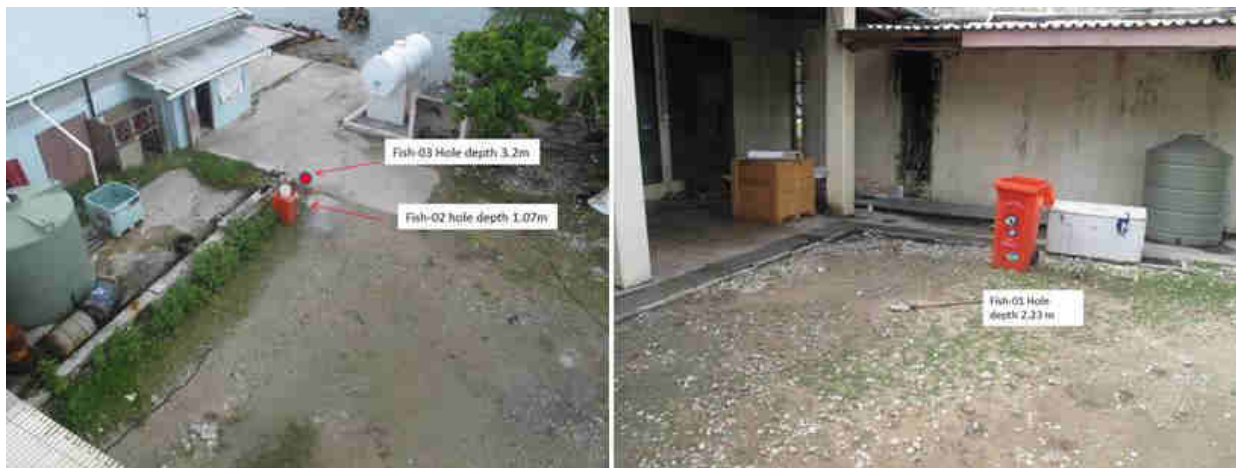
Figure 30 – Drill hole locations in the courtyard of the Fisheries Department, Fongafale. On the left, drill holes Fish-02 and Fish-03 were drilled. Drill hole Fish-03 was drilled through the concrete which help support the upper part of the hole. Drill hole Fish-01 was drilled adjacent to the room used as a library.
