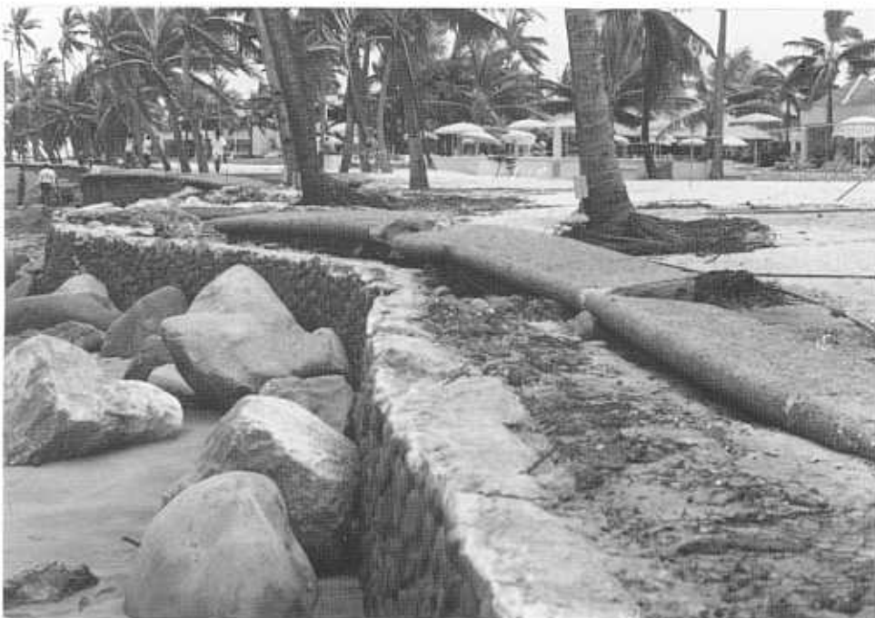
December 1990: Sheraton seawall - after Sina. Note buildup of sand fronting wall and removal of concrete capstones.
