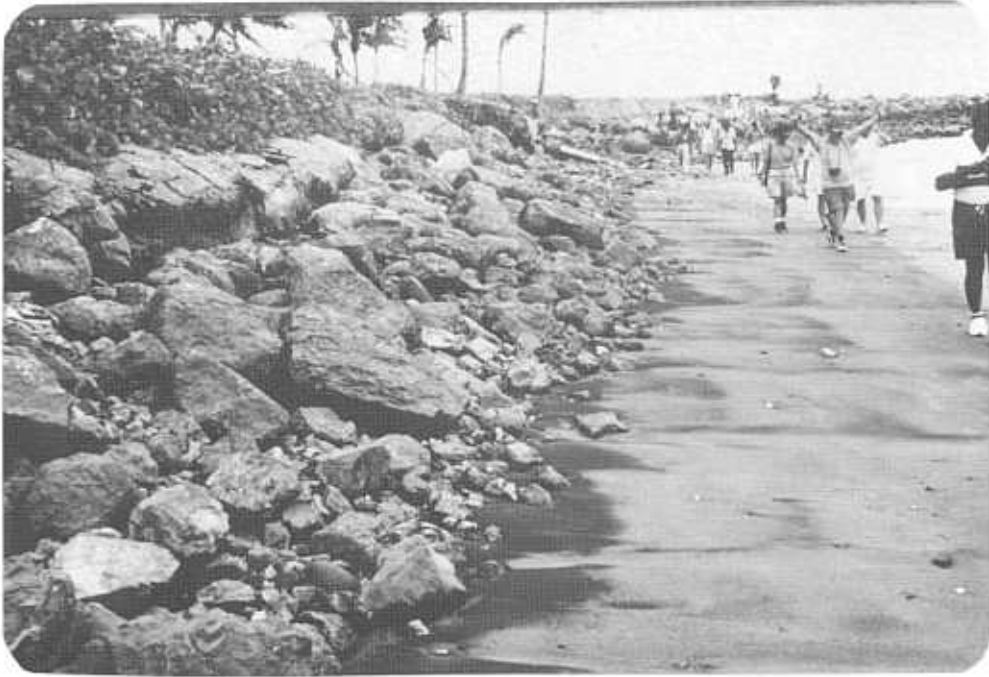
September 1990: Sheraton west side - before Sina. Note: poorly designed rubble mound protection.
