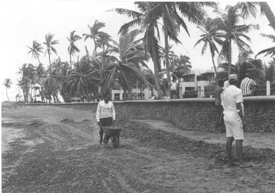
December 1990: Sheraton seawall - after Sina. Note buildup of sand fronting wall.
