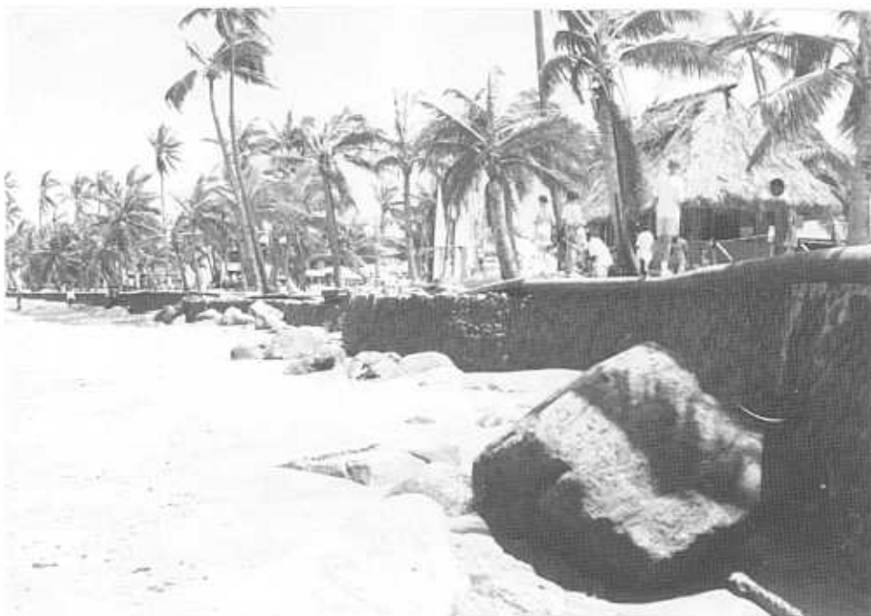
December 1990: Sheraton seawall - after Sina. Note the buildup of sand fronting wall.
