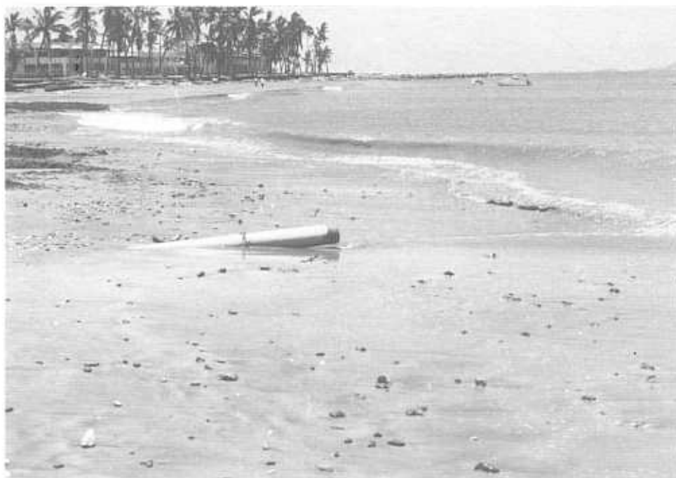
December 1990: Sheraton west side - after Sina. Note: outfall pipe near Regent Hotel is broken and spilling onto beach.
