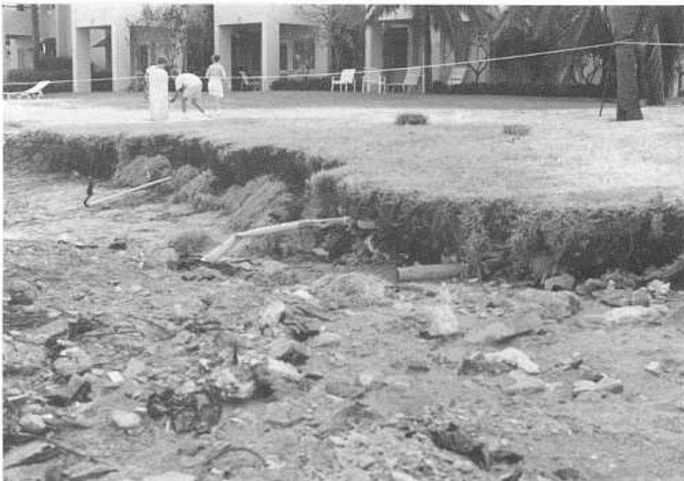
December 1990: Sheraton west side - after Sina. Note: erosion of lawn exposing irrigation pipes. Debris in bank indicates that this was reclaimed land.
