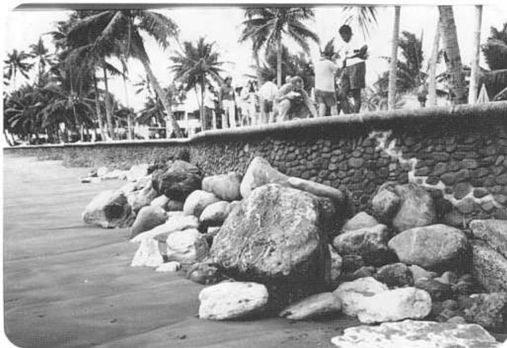
September 1990: Sheraton seawall - before Sina. Note: scouring of bottom step.
