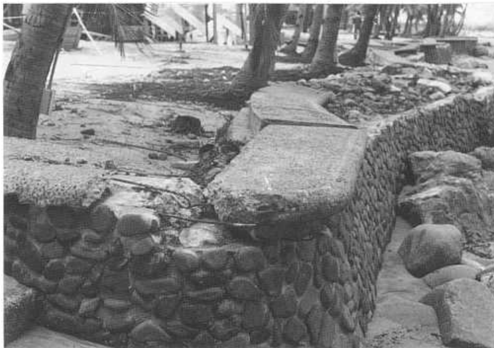
December 1990: Sheraton seawall - after Sina. Note: scouring and broken capstones.
