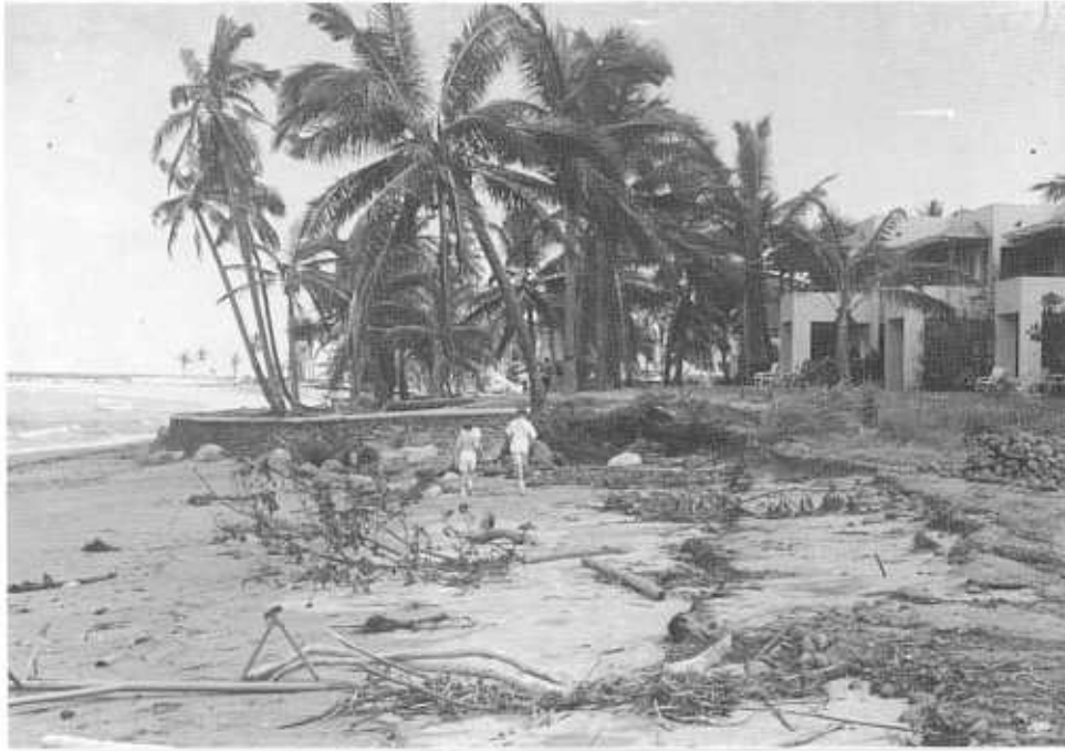
December 1990: Sheraton seawall - after Sina. Note scour around the east end of the seawall but the adjacent original natural beach slope is changed little.
