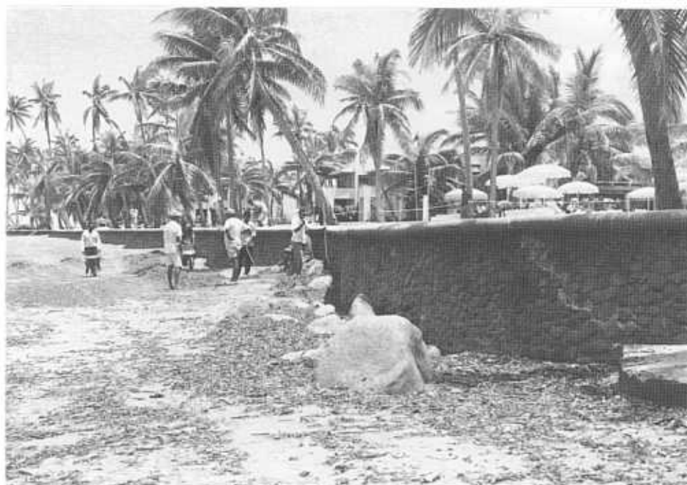
December 1990: Sheraton seawall - after Sina. Note: buildup (0.5 m) of sand at bottom step.
