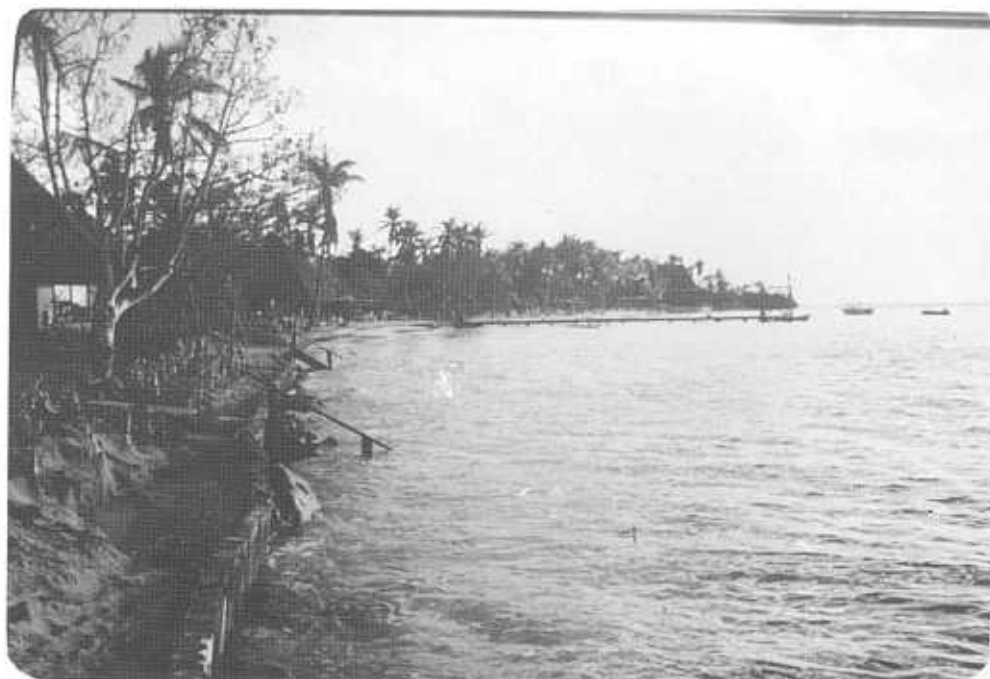
December 1990: Fijian Hotel - after Sina. Note: sand scoured from behind wall.
