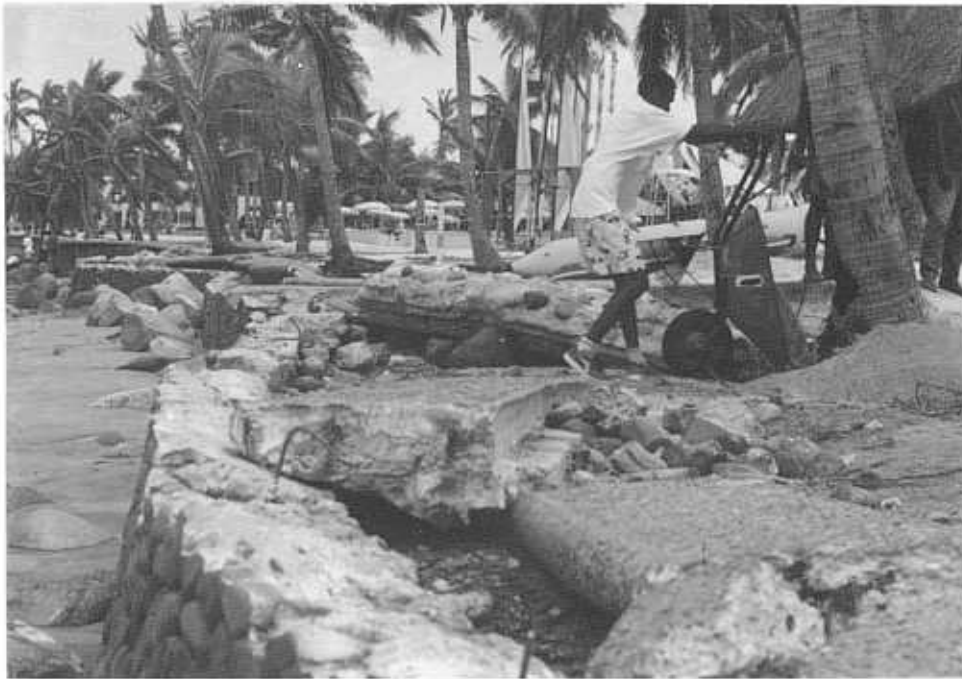
December 1990: Sheraton seawall - after Sina. Note: removal of concrete capstones and scouring behind wall.
