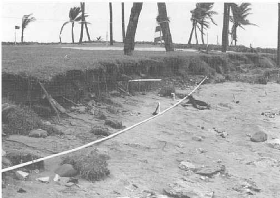
December 1990: Sheraton west side - after Sina. Note: irrigation pipes exposed and debris in bank indicating reclaimed land.
