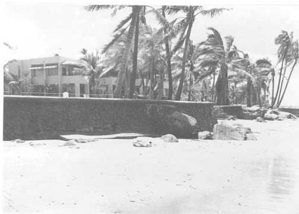
December 1990: Sheraton seawall after Sina. Note: sand buildup (0.5 m) flush with concrete slab and boulder (1 m diam.) upon concrete slab.
