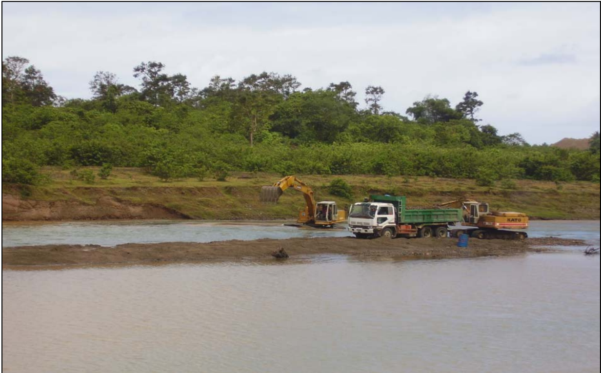
Figure 25. Excavator on the left is extracting aggregates from the opposite bank and passes it to the second excavator on the right for loading in the dump truck. Bank erosion is noticeable along the banks.
