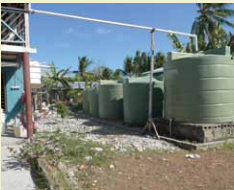
Rainwater tank farm, Funafuti, Tuvalu, 2011.
