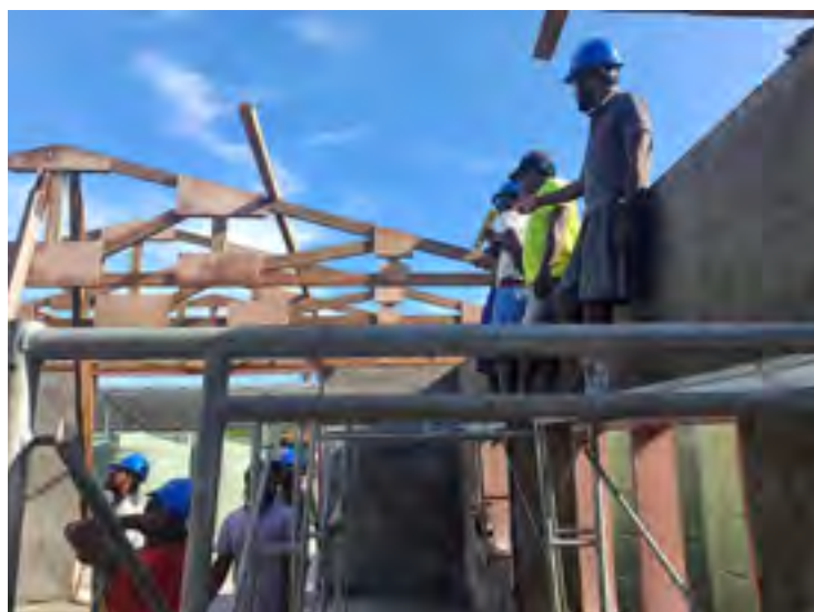
Construction in progress of new water facility infrastructure in Banaba Island, Kiribati
