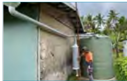
Household rainwater harvesting system, Niue
