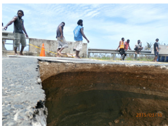
Collapsed bridge in Teoma, Efate Island, Shefa Province.
