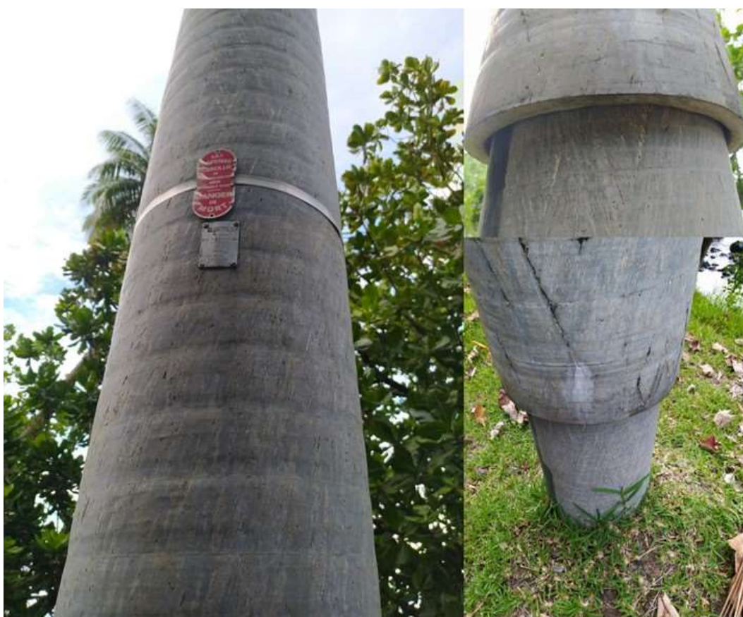
Photo 34. Poteau de ligne, fibre- ciment, Tahiti
