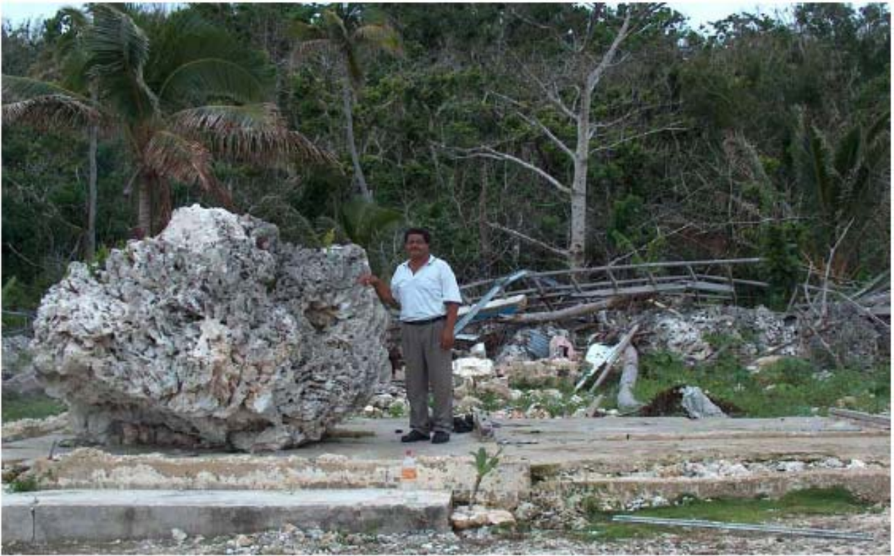
Figure 2: Deve Telagi, Director PWD, standing on the foundations of a destroyed building in Hikutavake and next to the biggest boulder picked up by the waves (~3-4 t). The boulder was thrown on the cliff edge during TC Ofa and during TC Heta transported some fifty metres further inland and smashed into this building.
