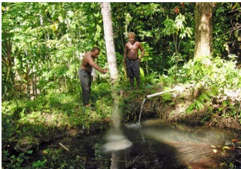
An experimental tilapia pond constructed on the initiative of Mr Fred Manu in 2002 in North Malaita, as a village-level development project. The growth rate of the tilapia was so slow that the project was suspended. This is because only Mozambique tilapia is presently available in the Solomon Islands. (Photo: Tim Pickering).
