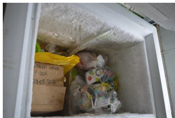
Figure 7 Solar powered deep freezer in Malekula
