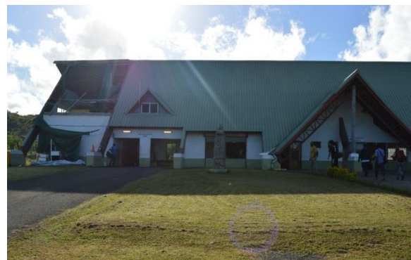
Figure 30 Tanna's Whitegrass Airport showing TC Pam damage to terminal building roof
