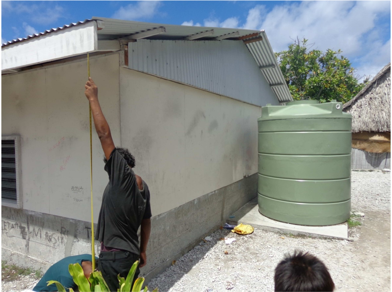
Figure A11-12. Survey team measuring the roof height of a private building in Rungata Village.
