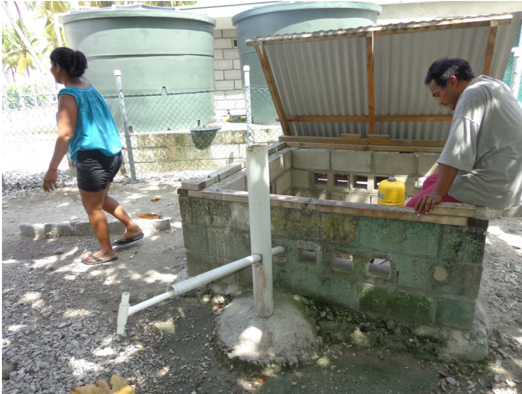
Figure 11. Locally-made Tamana pump or hand pump used for abstraction of groundwater from a nearby local well, Nikumanu, Nikunau.
