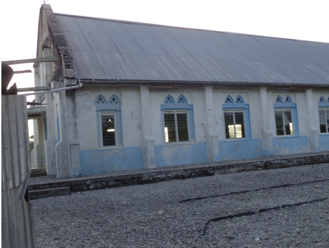
Figure A11-10. KPC Church in Nikumanu, a potential rainwater harvesting site for the village.
