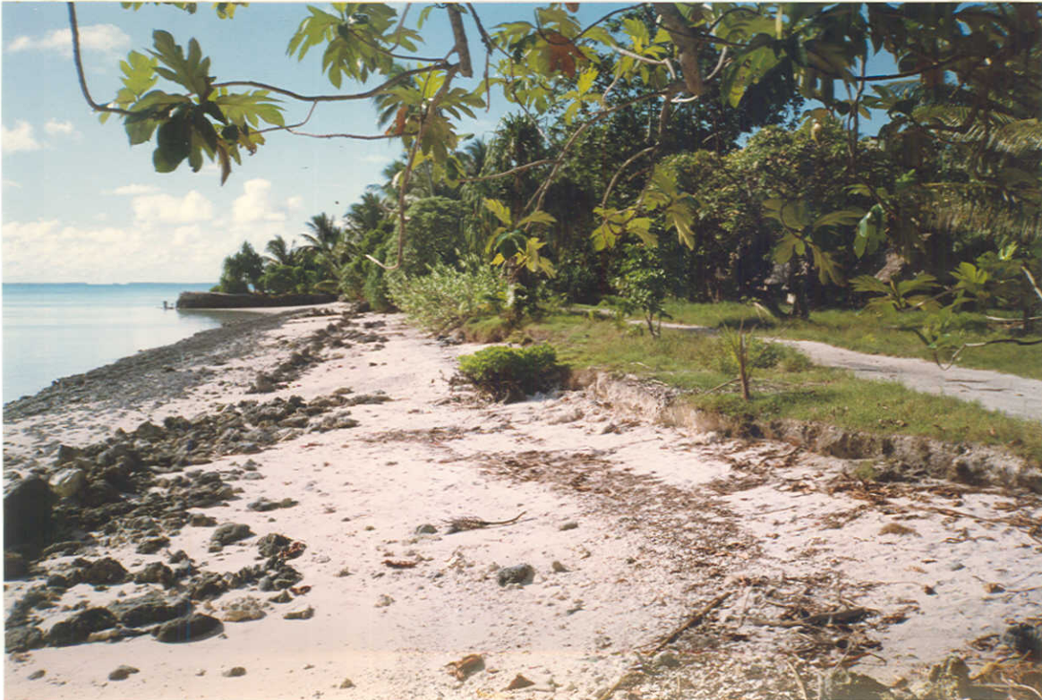
Figure 6. Koinawa, Abaiang. View north along lagoon shoreline showing remains of previous rubble mound seawall on beach. The main island road is located immediately behind the beach.
