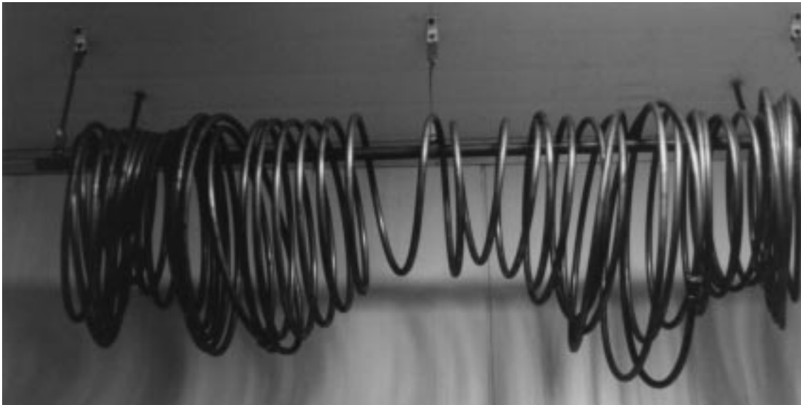
Figure 8: Copper piping mounted in chill room to provide chilled water to processing area
