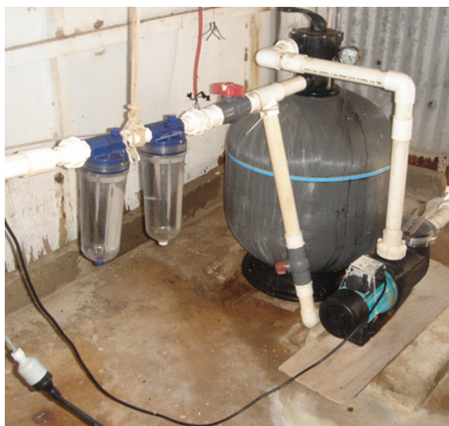
Water filtration system in a quarantine area
