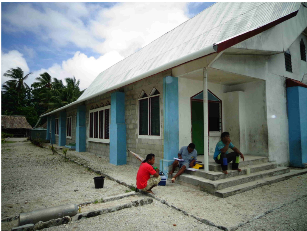
Figure A12-4: Ribono Catholic Church, a potential rainwater harvesting centre, with considerable infrastructural improvements needed.
