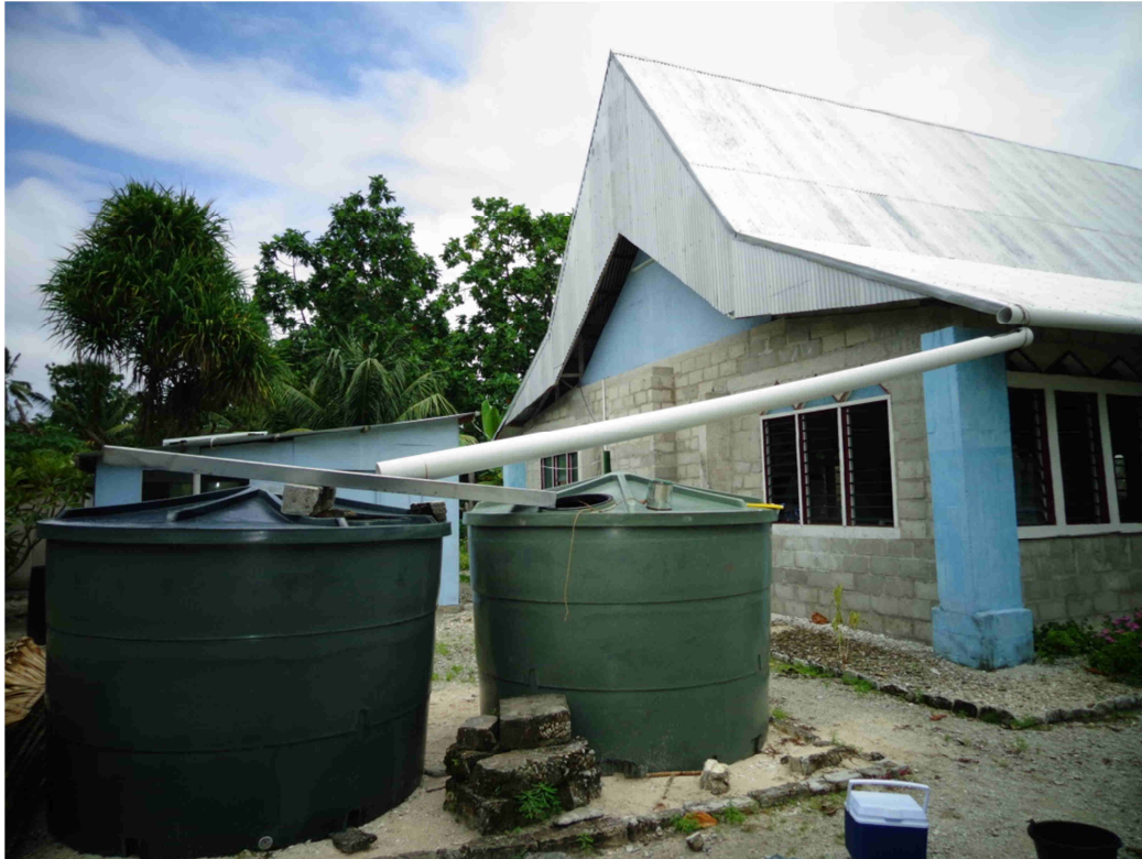
Figure A12-5. Two polyethylene tanks connected to the Ribono Catholic Church roof catchment, which has around 50 % guttering coverage.
