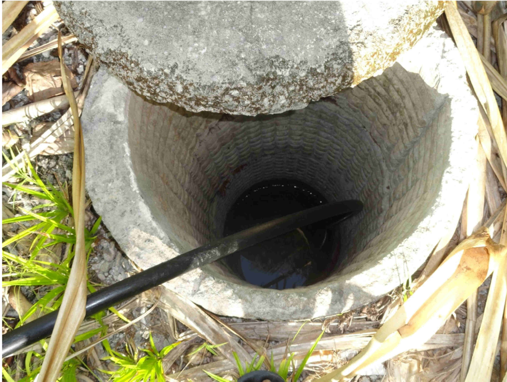
Figure A12-9. Household well using concrete rings and concrete lid and a poly-pipe connected to a pump – the well can be improved by installing concrete aprons.
