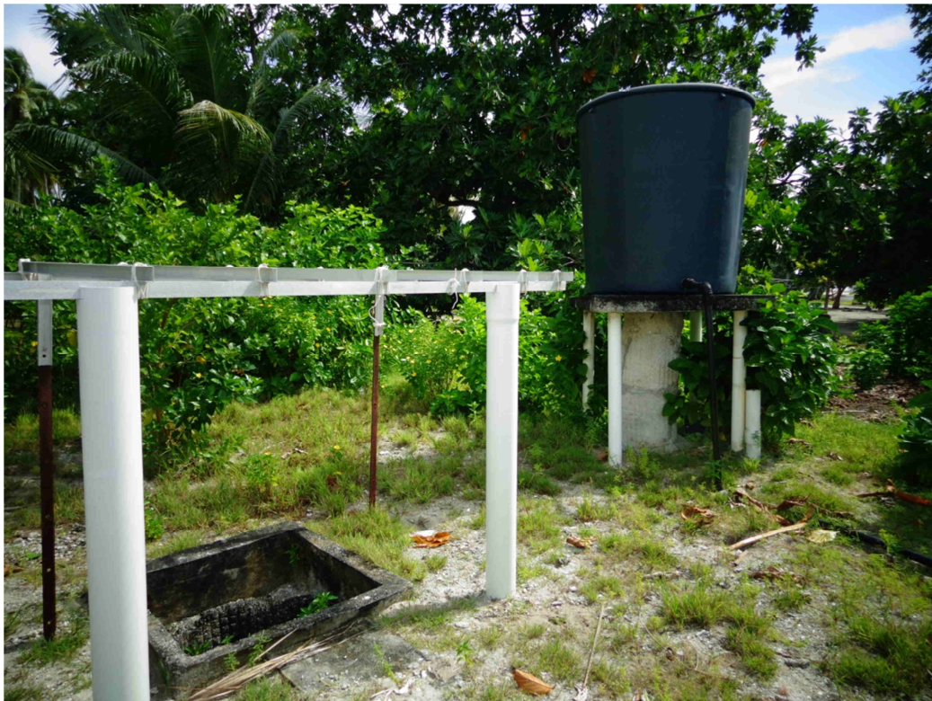
Figure A12-6. The Ribono Primary School well, which was reported to have a damaged submersible pump and stolen solar panels. Elevated 2,000 L polyethylene storage tank, in a good condition.
