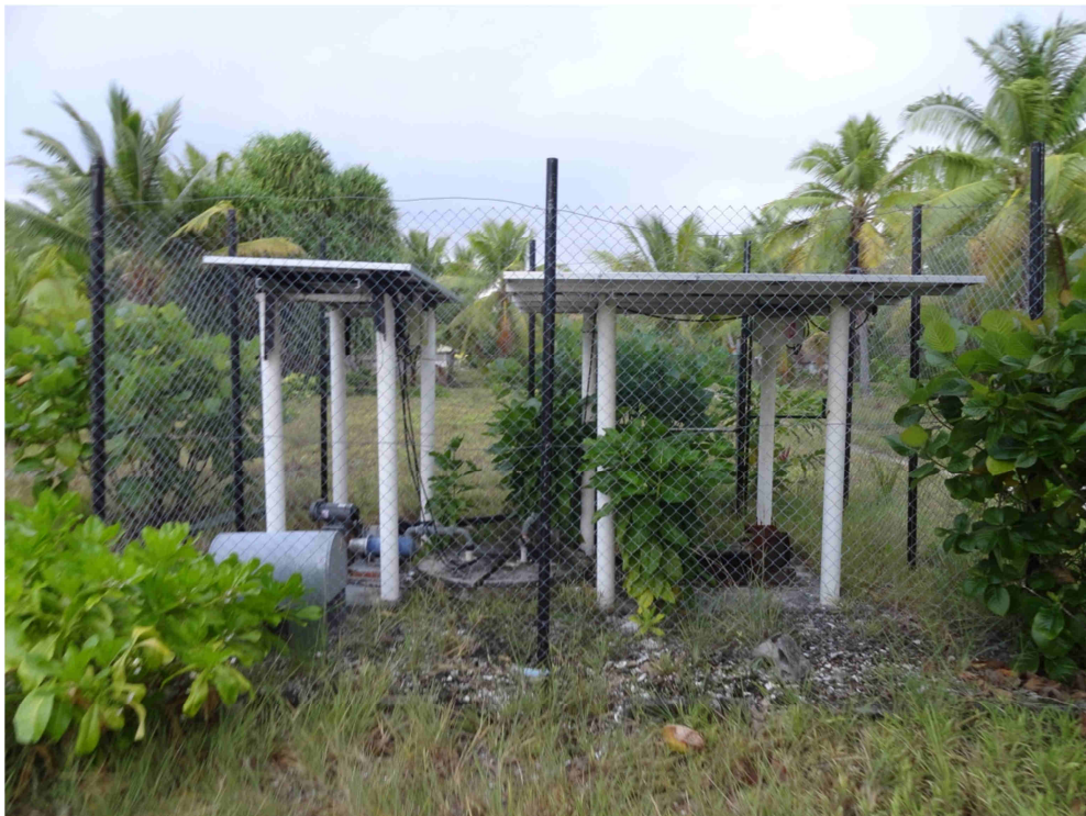
Figure A12-12. Solar pump system serving the entire St Joseph College school community, including the classrooms, hostels and staff quarters. There are reports that the well capacity is insufficient for the current demand and experiences elevated salinity during dry periods.
