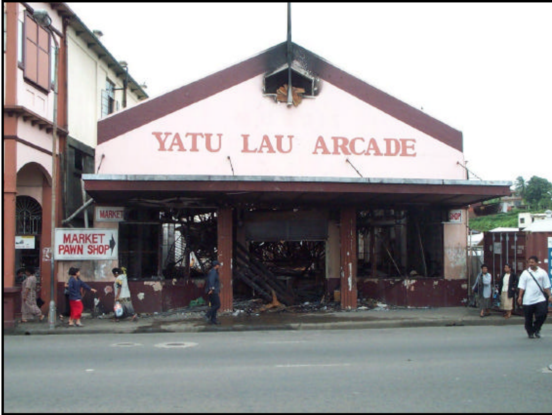
Figure 7a. Yatu Lau Arcade – A severely Damaged Building
