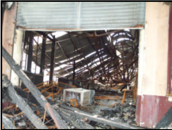
Figure 7b. Burnt Debris Blocks the entrance to Yatu Lau Arcade
