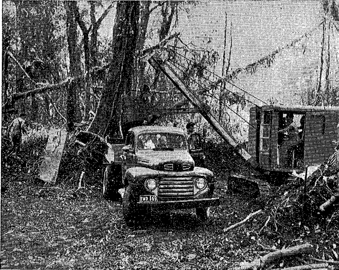
A Public Works Department mechanical shovel quarrying scoria at the roadside for road building.
