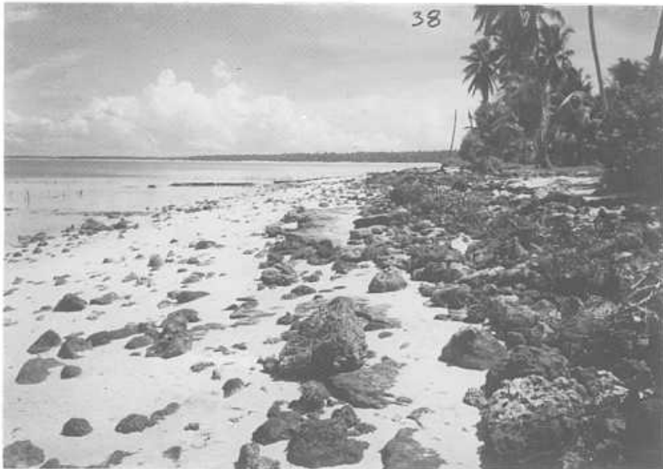
Figure 8. Collapsed gabion seawall, south of Tebunginako maneaba. Shown as Figure 27 in Harper 1989.
