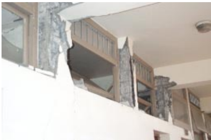
Figure 21: Short columns spalled and failed, ground floor, Lycee Bougainville.
