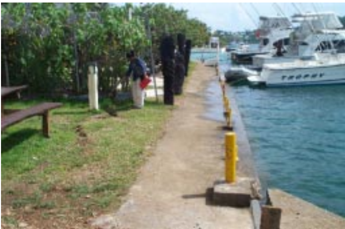
Figure 30: Ground fissures and tilted sea wall near Waterfront Bar.
