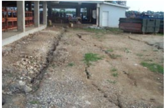
Figure 27: Fissuring in back-fill behind sea wall, north of Market.
