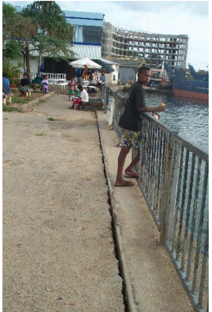
Figure 31: Gap between sea wall and back-fill.
