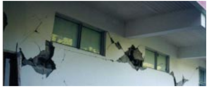
Figure 26: Damage at the Imford Museum.
