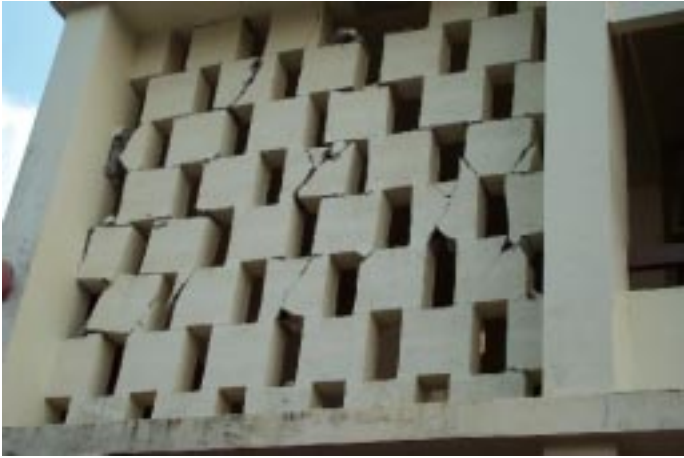
Figure 24: Infill block-work in stairwells of the Lycee Bougainville sheared and collapsed.
