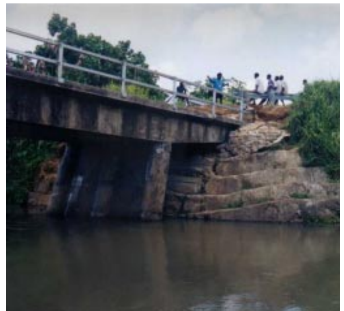
Figure 33: Damaged Teouma Bridge, eastern abutment.
