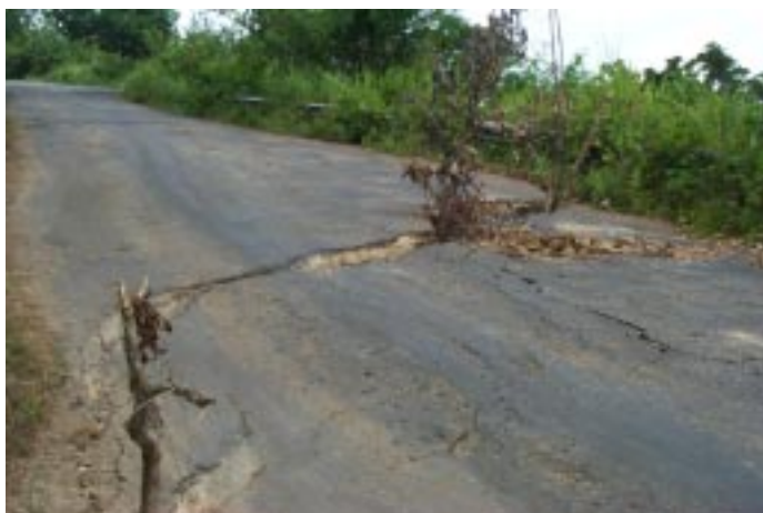
Figure 45: Transverse fissures on Efate ring road at Klem's Hill.
