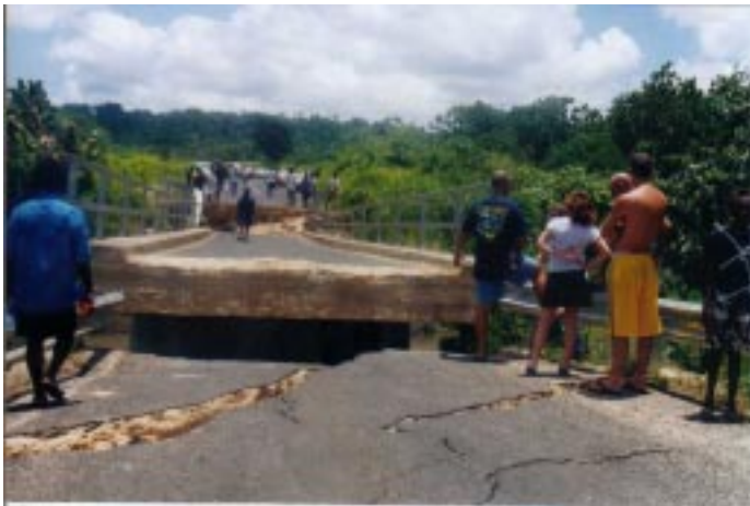
Figure 34: Damaged Teouma Bridge, western abutment.
