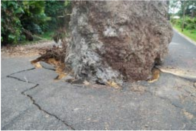
Figure 39: Toppled limestone boulder puncturing surface of the main Star Wharf access road.
