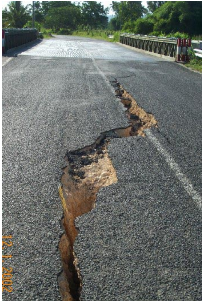
Figure 37: Embankment failure, Prima Bridge.
