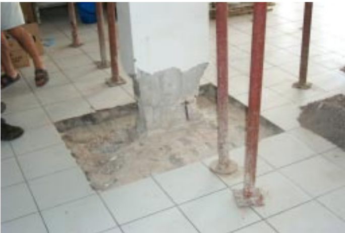
Figure 25: Damage around ground-floor columns at Au Bon Marche.
