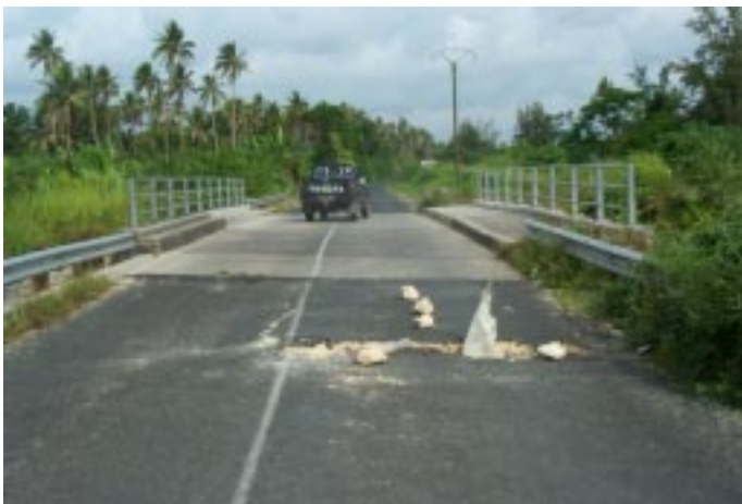
Figure 35: Embankment failure, Mele Bridge.
