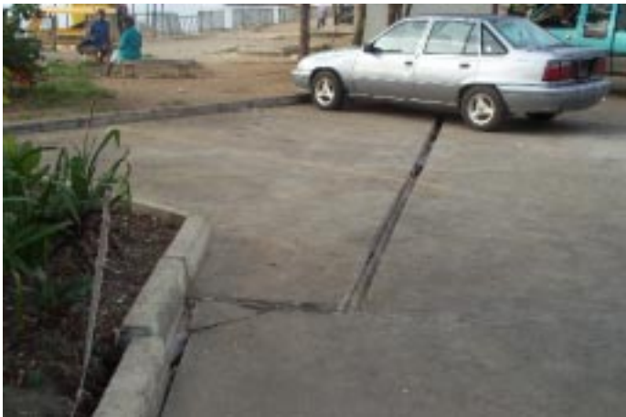
Figure 29: Car park slabs opened on construction joints south of Market.
