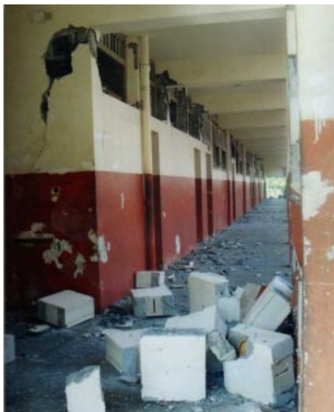
Figure 23: Damage to ground-floor classrooms of the Lycee Bougainville.
