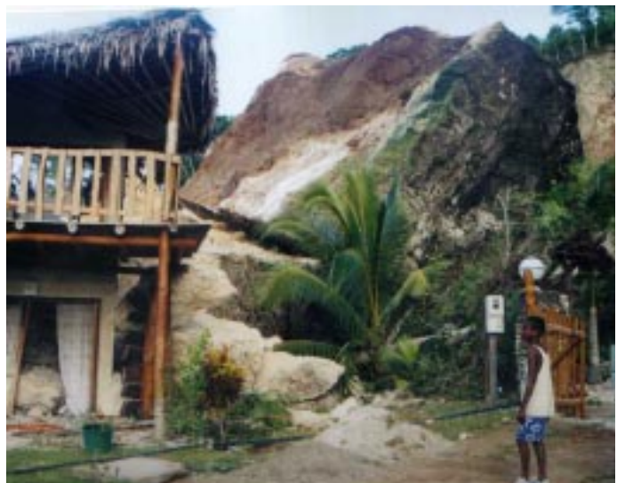
Figure 44: Bungalow damaged by rock-fall at Pango resort.
