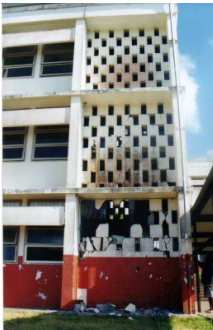
Figure 22: Differential damage between upper and lower floors of the Lycee Bougainville.
