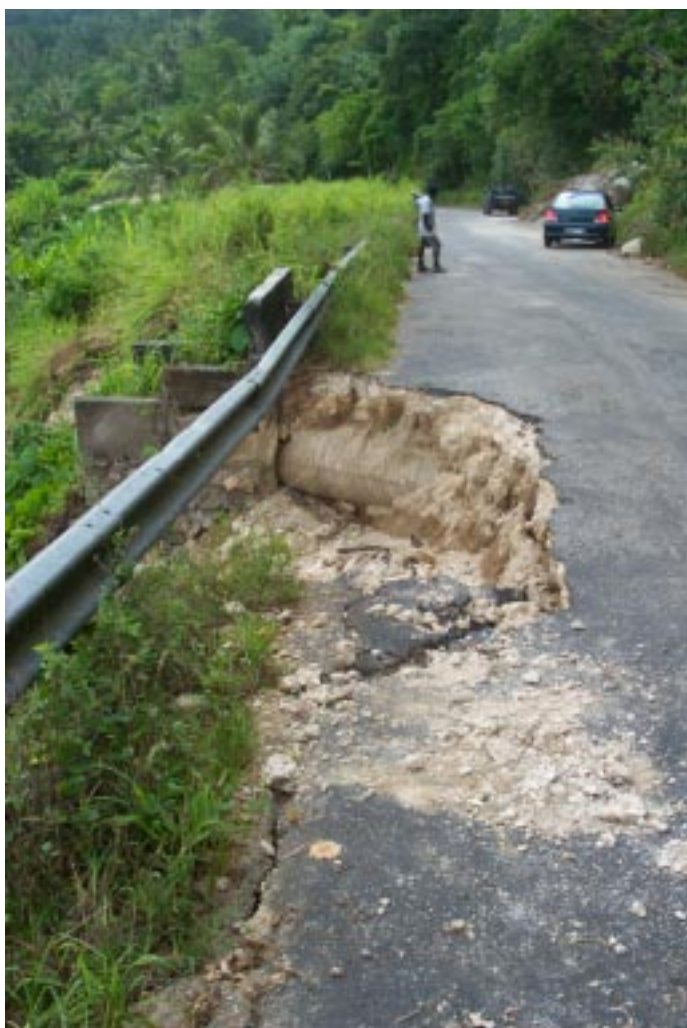
Figure 46: Landslide on Efate ring road at Klem's Hill.
