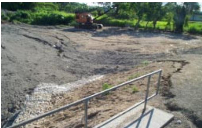
Figure 36: Slumping due to liquefaction, Prima Bridge.
