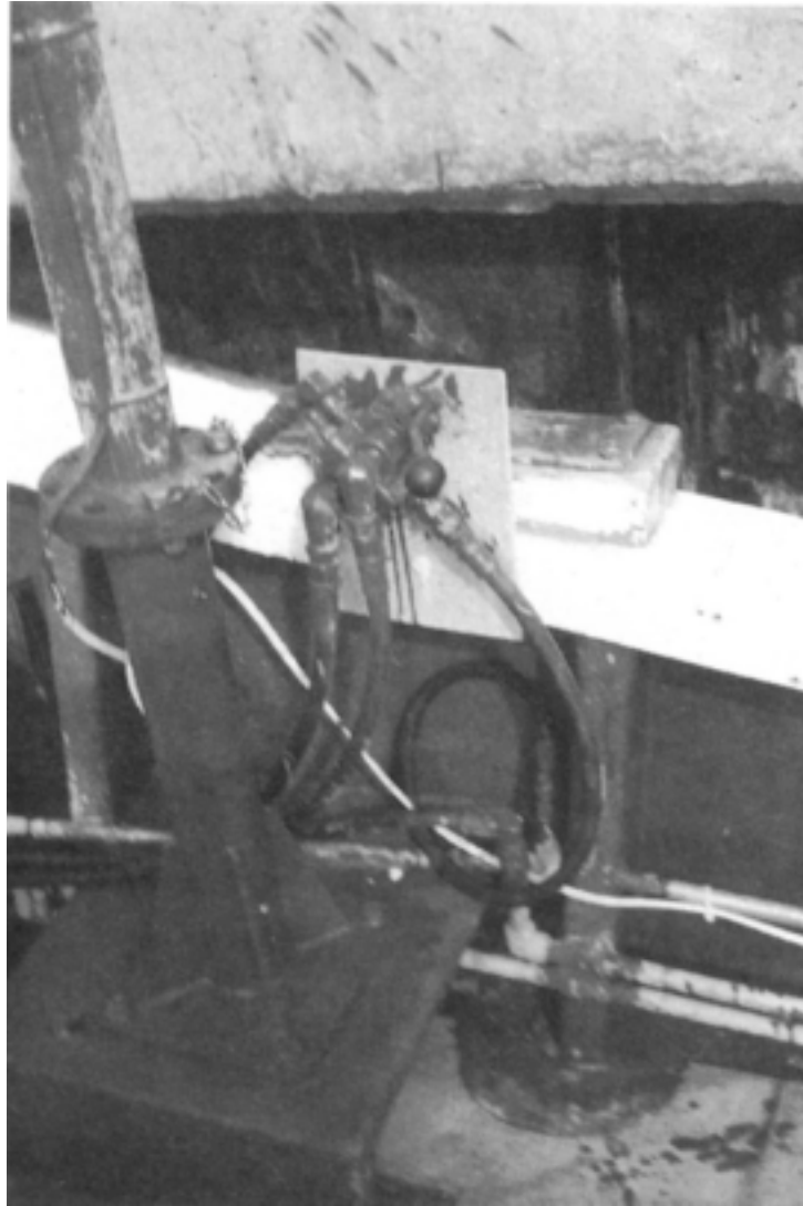
Figure 23: Hydraulic control valve for the longline drum mounted on the starboard rail
