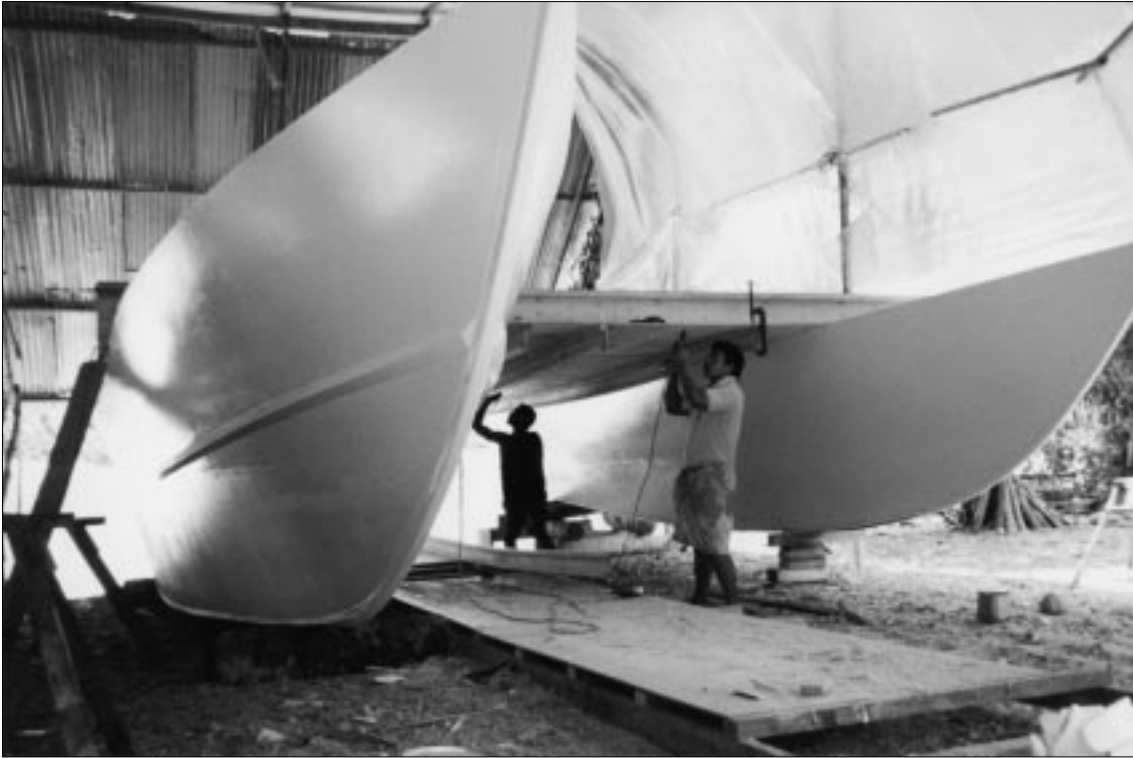
Figure 4: Hulls of the new twin-hull vessel being built in Kiribati with the deck being secured
